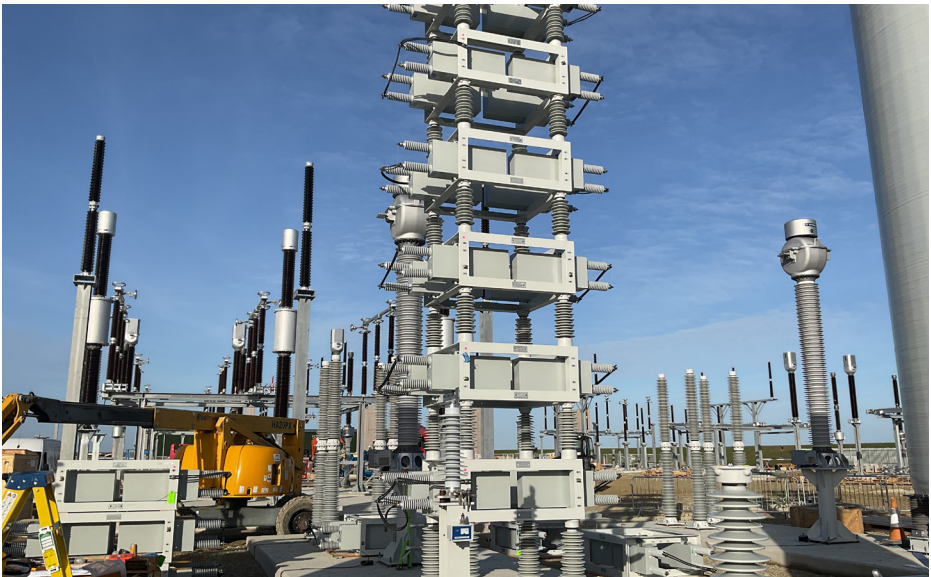
Harmonic filter in electrical compound.
