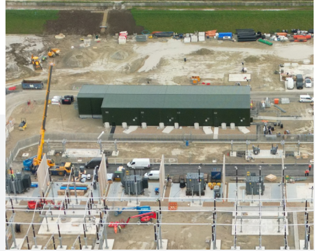
Switch room (green building) and transformers.
