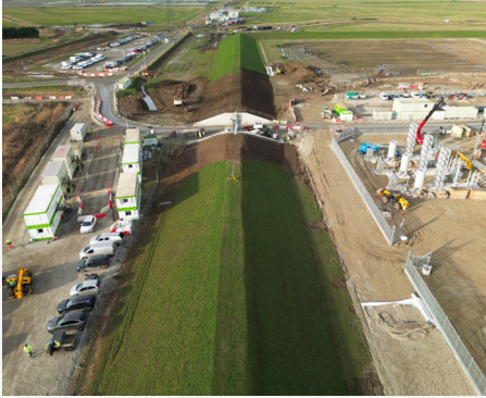
Protective bund surrounding electrical compound and flood gate.
